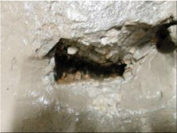
Bathurst – Waterproofing Foundation Wall Found active leak
