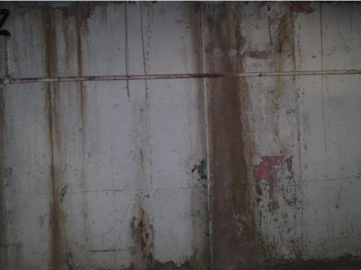
Bathurst – Waterproofing Foundation Wall Before – Evidence of water infiltration
