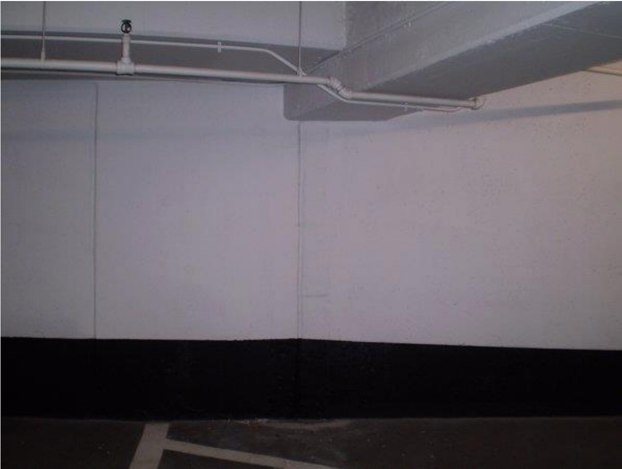
Brookfield – Waterproofing Construction Joints Painted finish – Looks brand new, in and out in four hours
