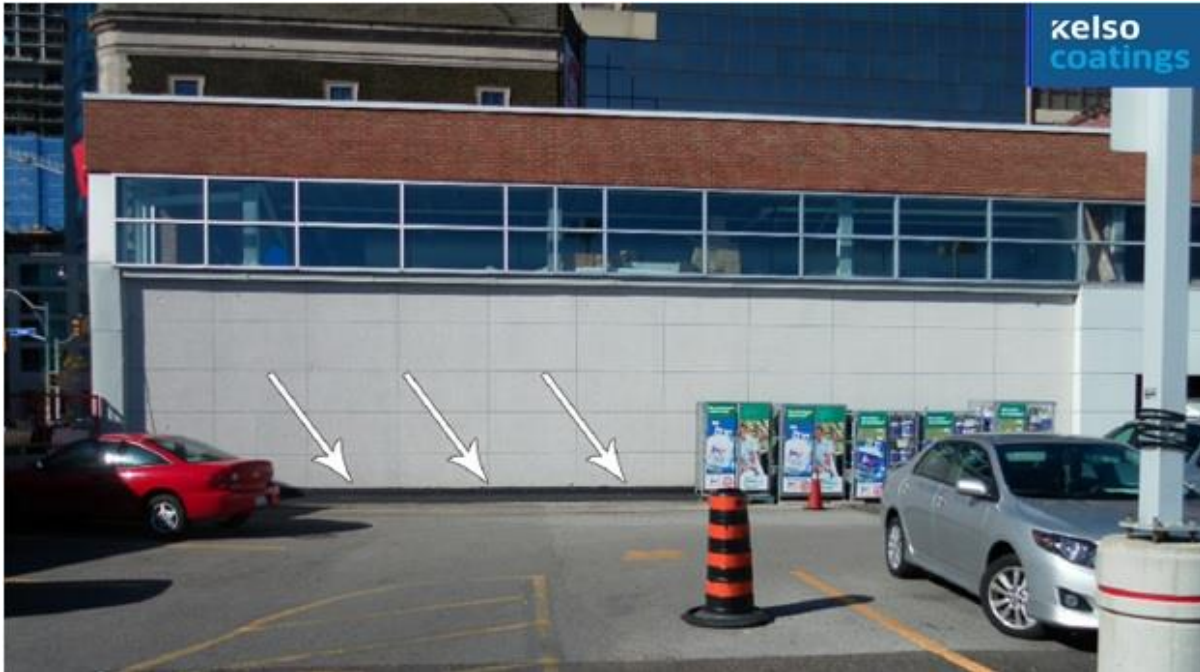
Canadian Tire, Toronto, Ontario Structural steel beams corroded due to water leakage
