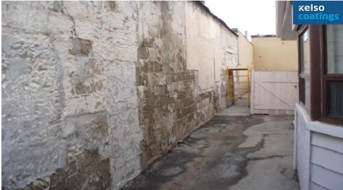
Midas Auto Service, Toronto, Ontario Water leaking through above grade foundation wall in hard rain
