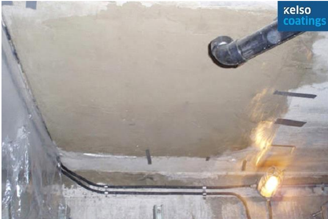
Toronto Transit Commission Station, Toronto, Ontario Major ceiling leak in electrical room
