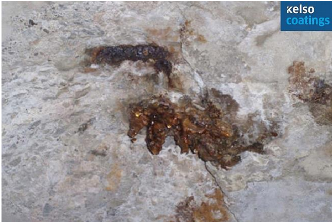
Toronto Transit Commission Station, Toronto, Ontario Major ceiling leak in electrical room
