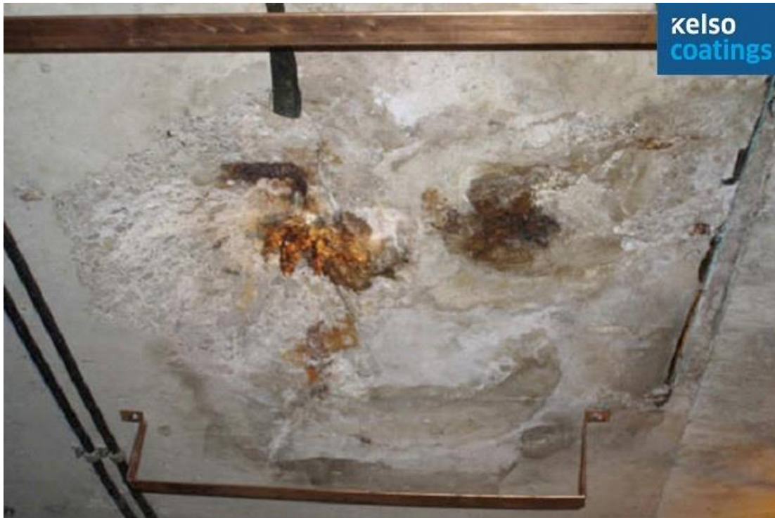
Toronto Transit Commission Station, Toronto, Ontario Major ceiling leak in electrical room
