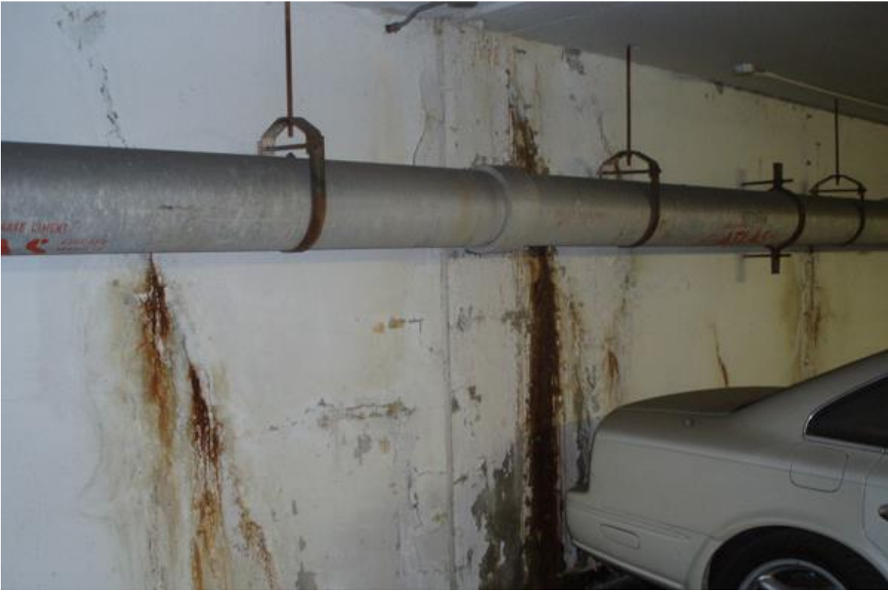
Townsgate – Failed injection wall
