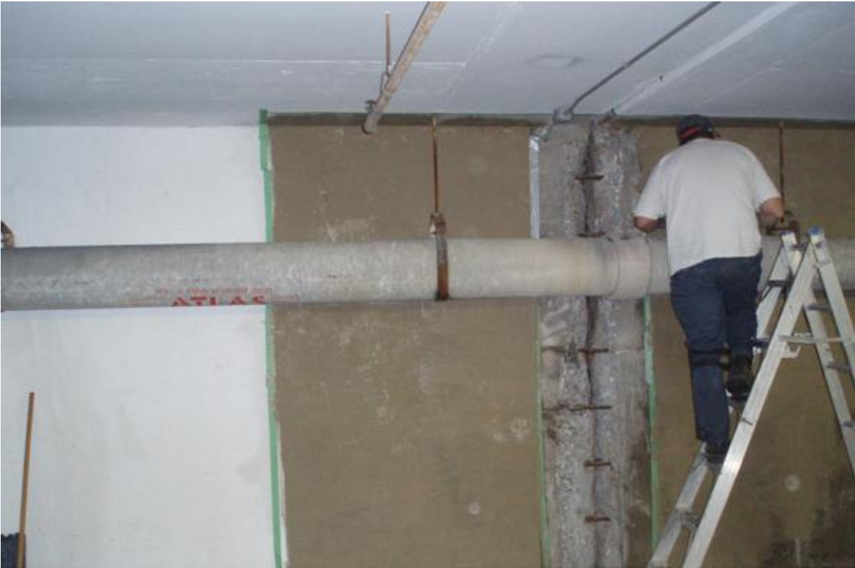
Townsgate – Failed injection wall
