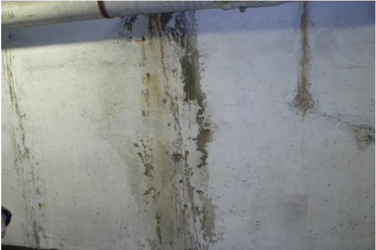
Townsgate – Foundation wall waterproofing Close view of cracks
