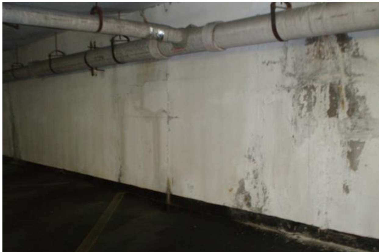
Townsgate – Y pipe
