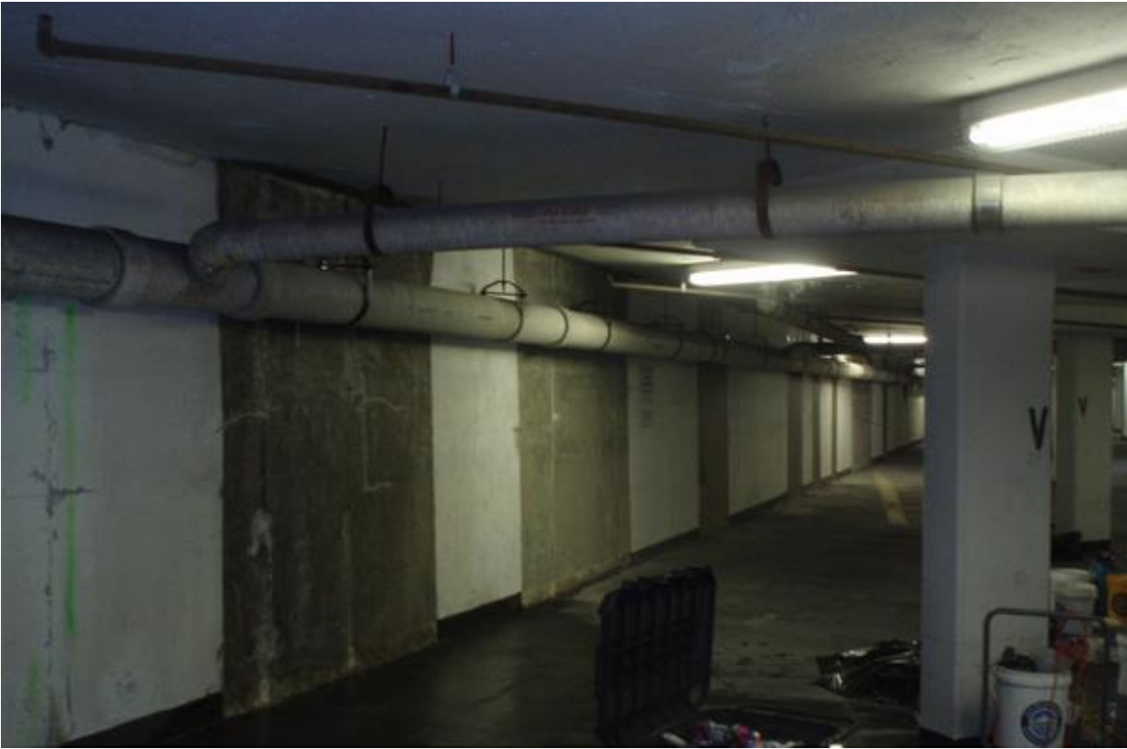
Townsgate – Y pipe
