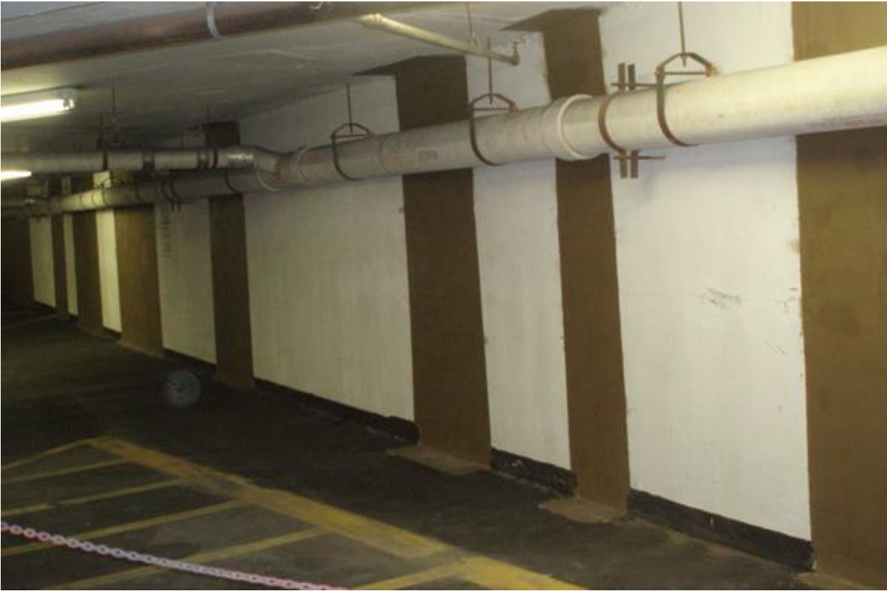
Townsgate – Y pipe
