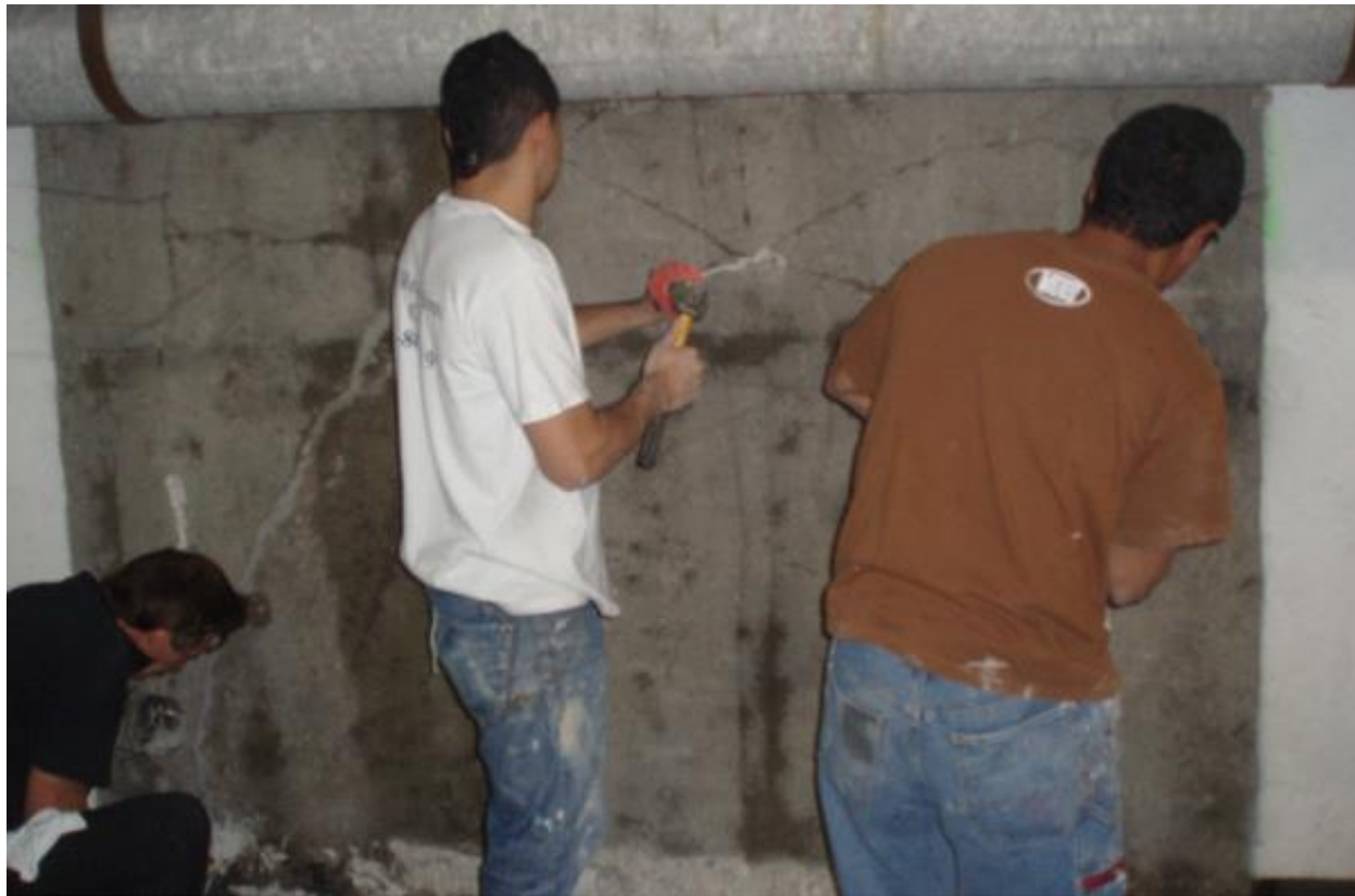
Townsgate – Y pipe
